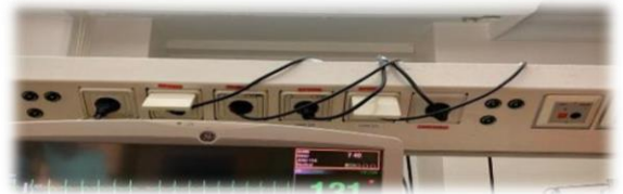
(Figure 2): Cables looped around the ceiling-mounted panel.
