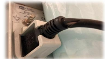
(Figure 3): Visible cuts on power cables
