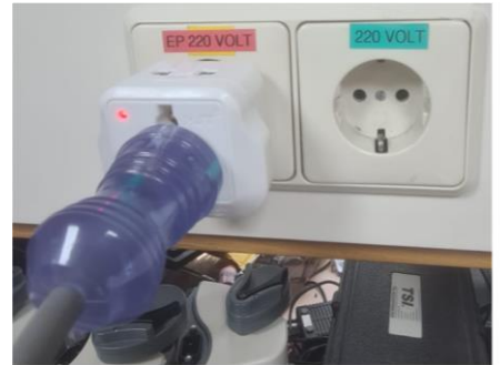
Figure 1 A 110V equipment forced to plugged in 220V outlet by using power adapter
